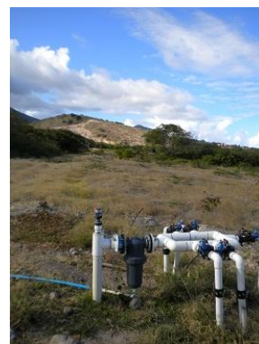
Irrigation System (Mar, 2011)
